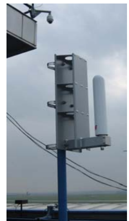
THALES ATM AS-680 Dispatcher TIS-B Transmitter
